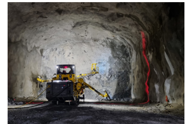
Extension work on the Stockholm Metro Blue Line from Gullmarsplan station. Sweden.
