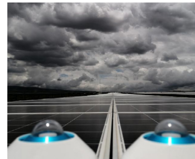
Perote photovoltaic solar plant. Mexico.
