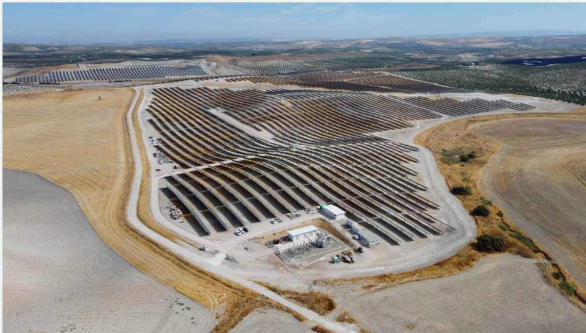
50 MW photovoltaic plant, Olivares, Jaén, Spain.
