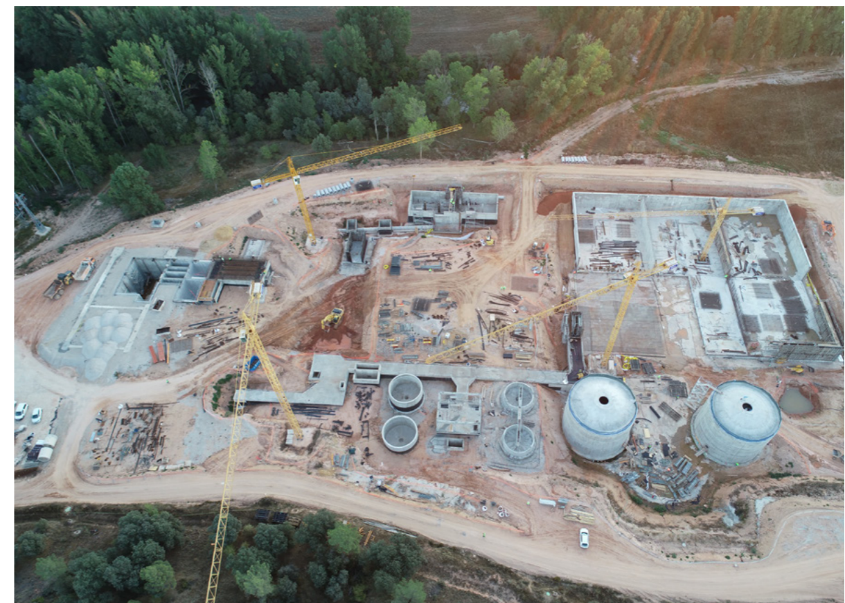
Sinova wastewater treatment plant. Soria, Spain.
