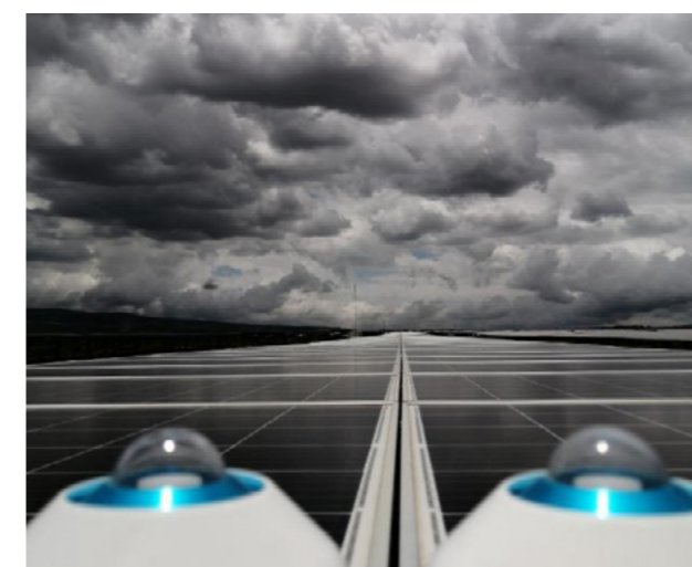
Perote photovoltaic solar plant. Mexico.
