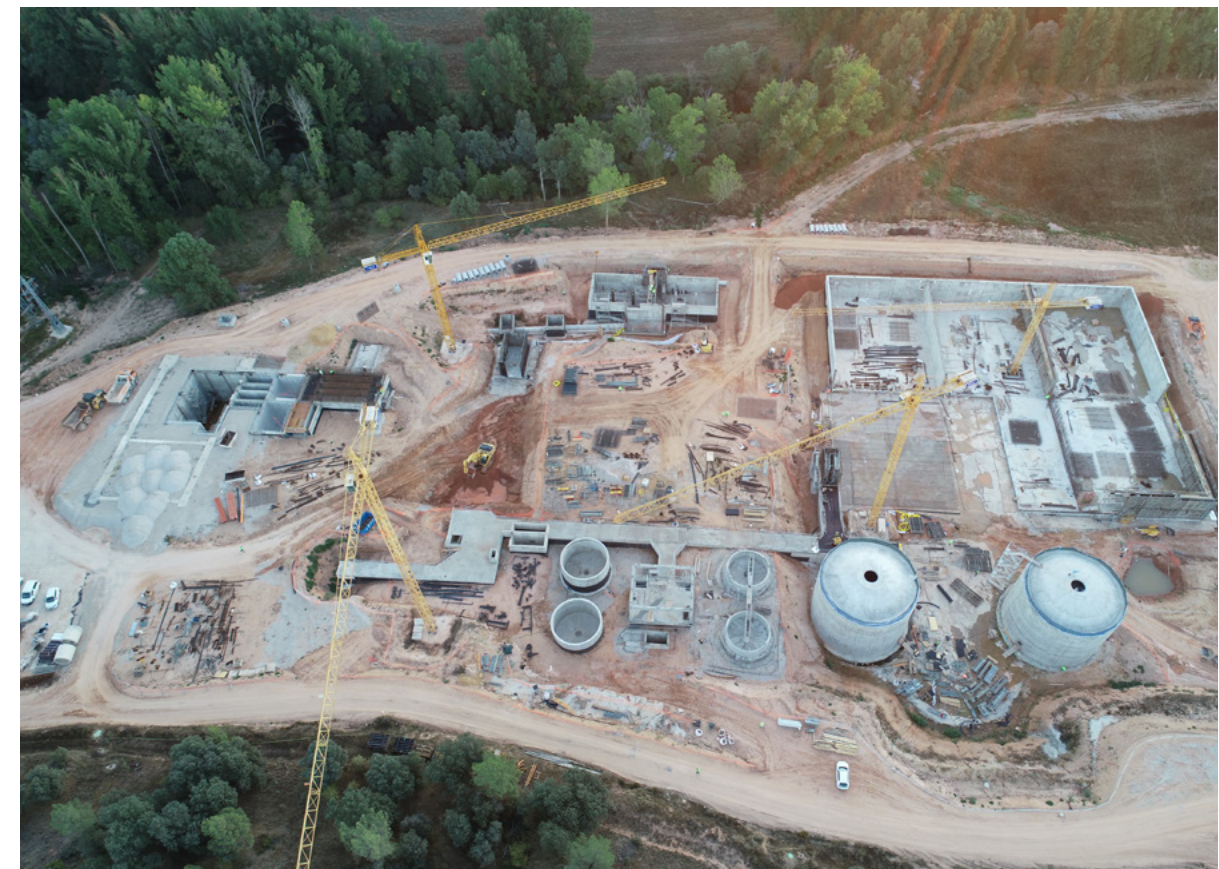
Sinova wastewater treatment plant. Soria, Spain.
