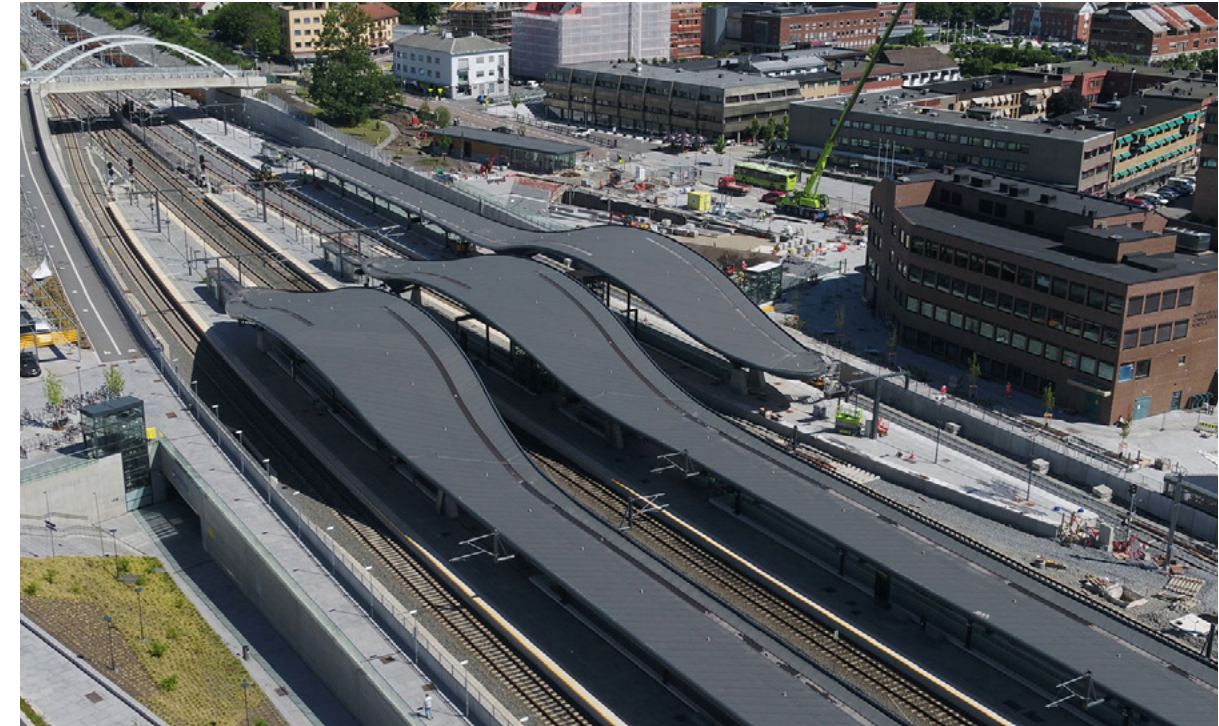
The Ski Project rail works, a part of the Follo Line. Norway.
