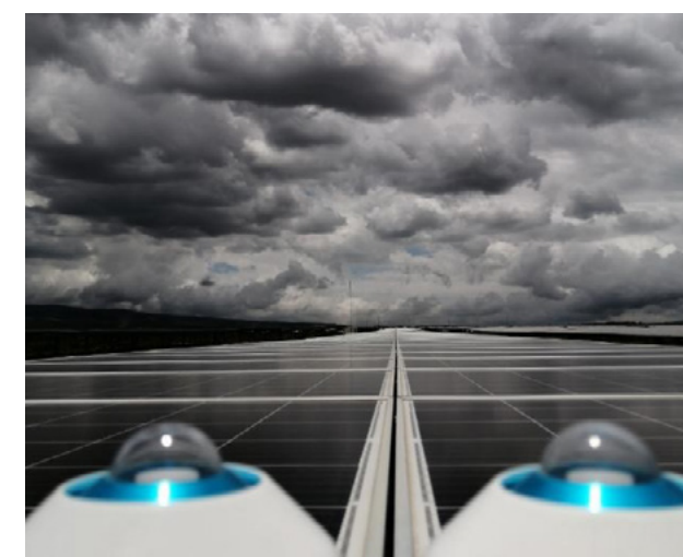
Perote photovoltaic solar plant. Mexico.
